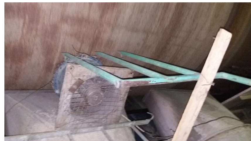
Rotary Kiln cooling
