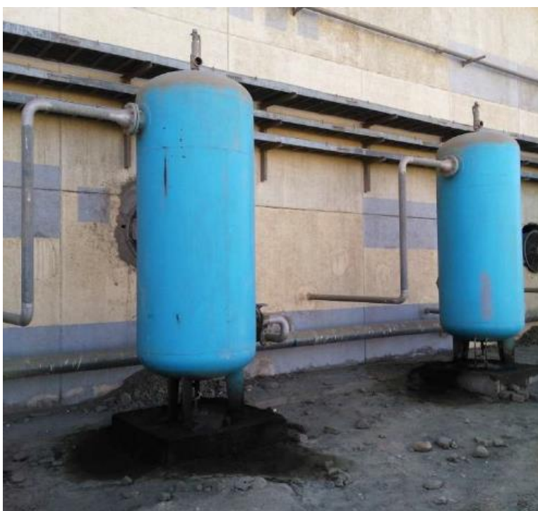
Figure 14-29: Receiving tank and drain system
