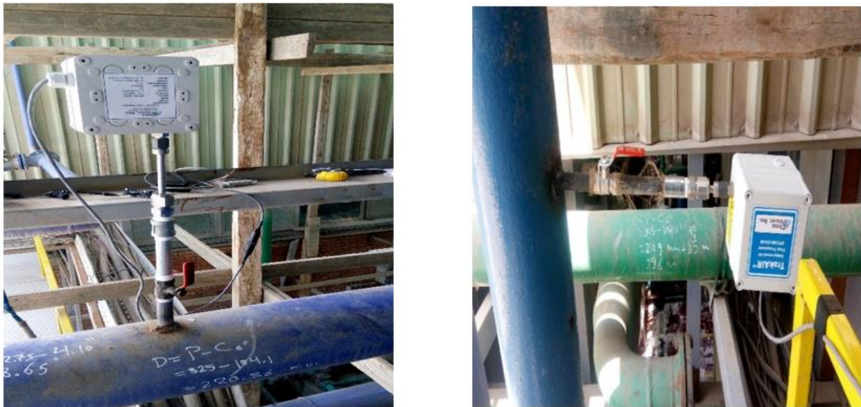
Figure 14-9: Air flow transducers at main feeder (left) and at LP pipe (right)
