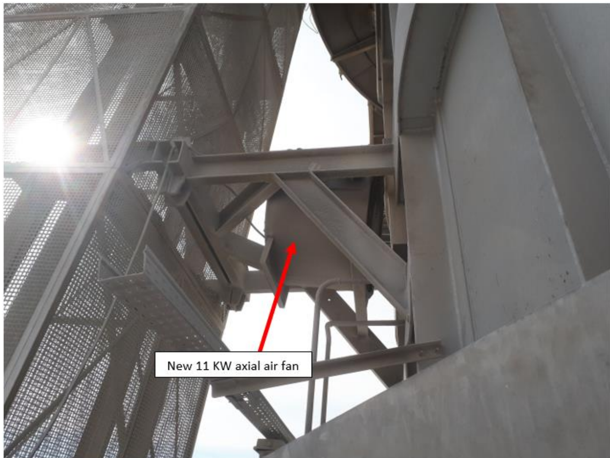
Figure 14-20: Lime plant shaft furnace with new air fan installed (after remedy action)
