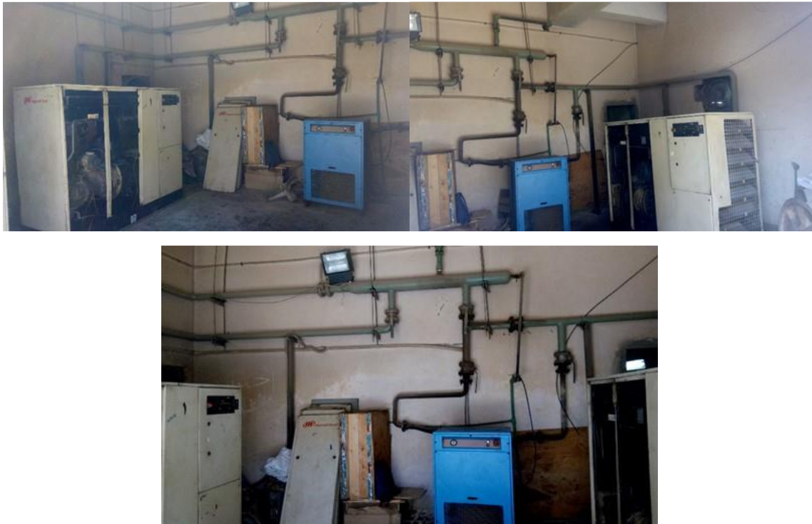
Figure 14-47: Furnace zone compressed air system
