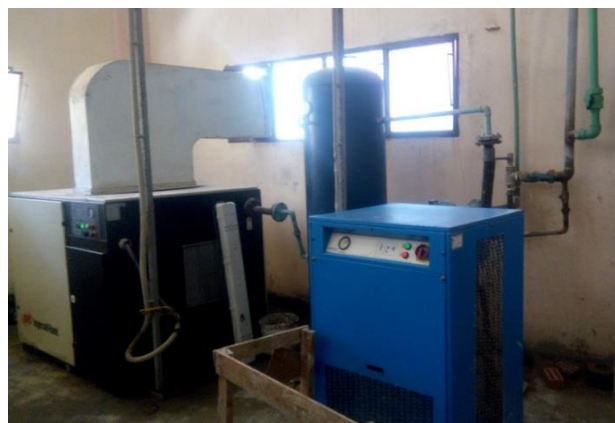
Figure 14-48: Liquid zone compressed air system room 2
