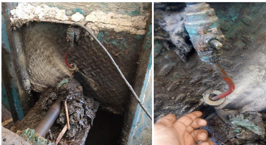
Figure 14-55: Inappropriate use of compressed air (Bearing cooling)
