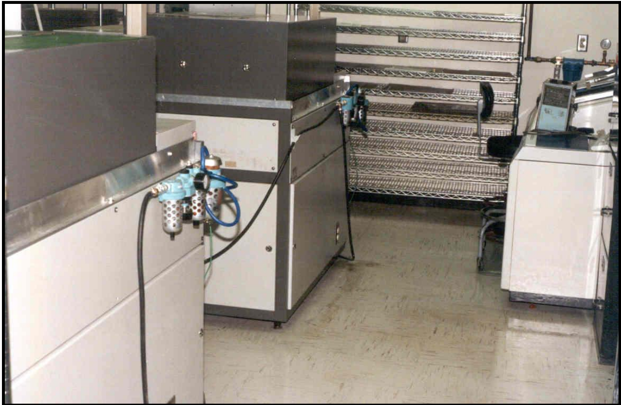
Figure 6-3: Test Machine Compressed Air Point of Use Connection
