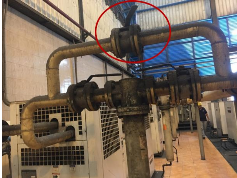
Figure 14-62: Partially open filter bypass
