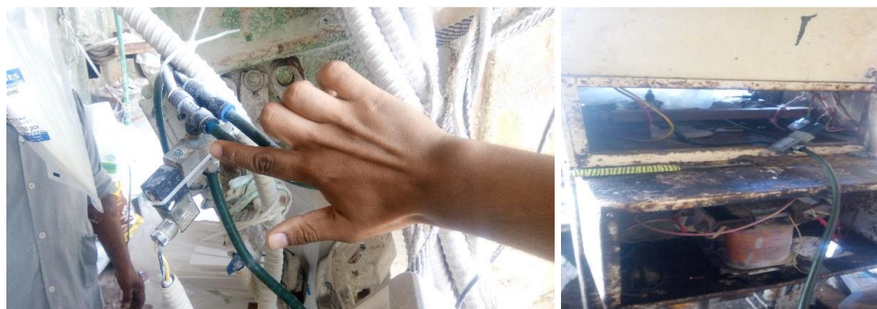
Figure 14-54: Examples of identified leak points on the demand side
