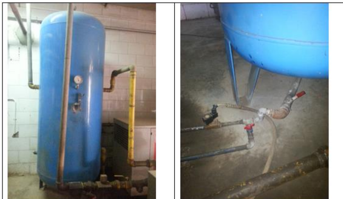
Figure 14-31: Receiver tank and drain system
