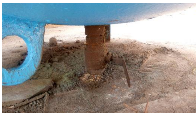
Figure 14-53: Tank Drain Valve
