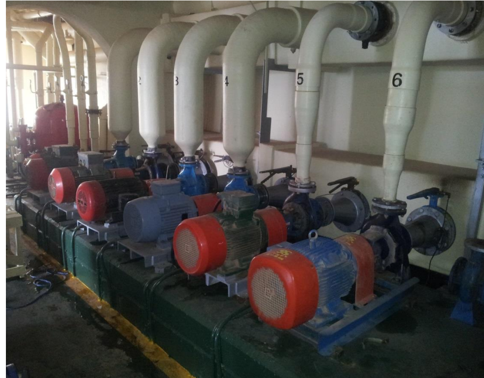
Multiple pumps in parallel
