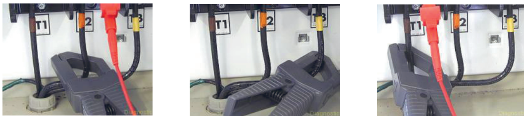
Fig. 12.28. Monitoring all Three Phases
