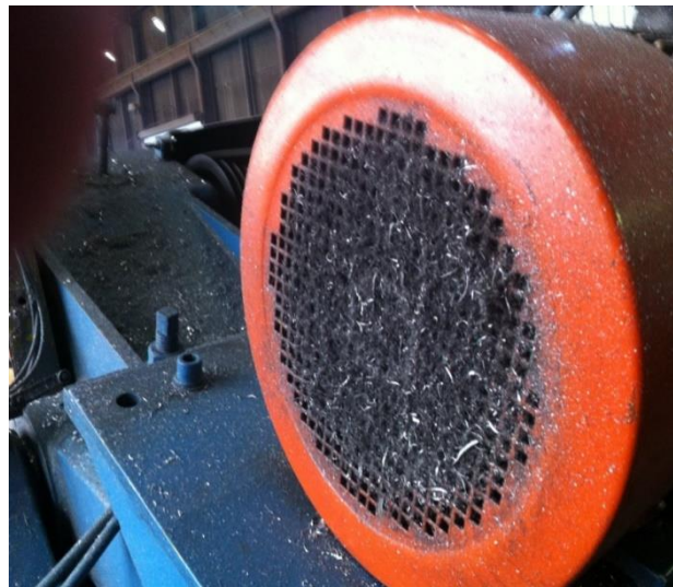
Figure 73 Partially blocked fan on an induction motor in a metal processing plant. (Atkins)
