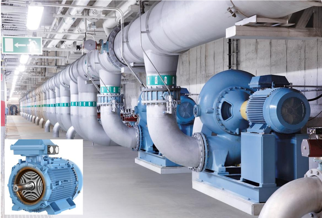
Figure 21 Pumping station using Synchronous Reluctance Motors (source:ABB)
